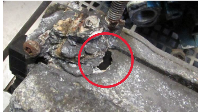
Holes in ECU cover
