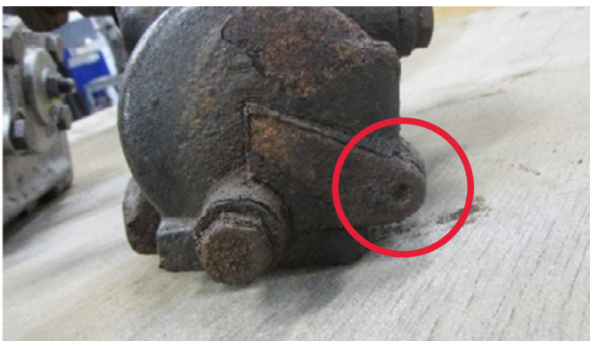
Improper process – damaged housing
