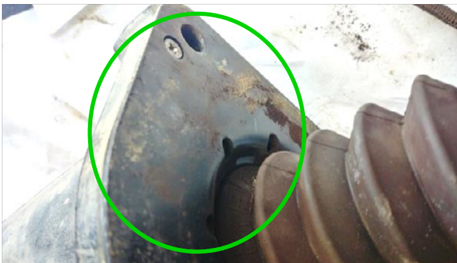
Dirt or corrosion on flange
