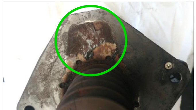
Dirt or corrosion on flange
