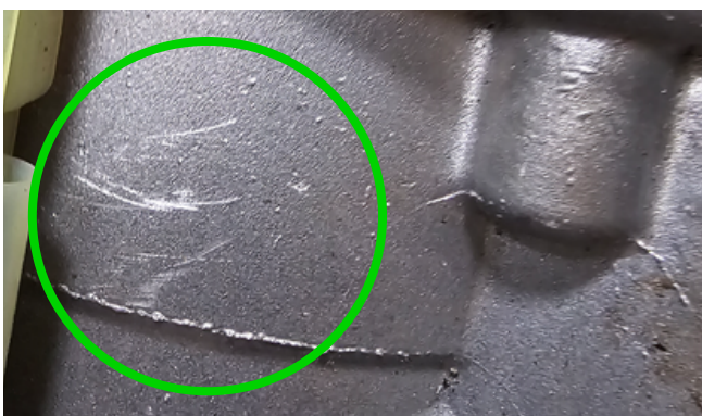
Scratches on external surface
