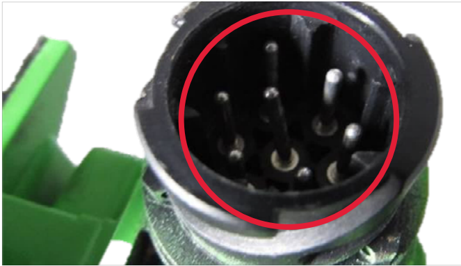
Missing, bent pins or corrosion in the connector
