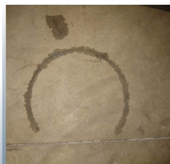
Evidence of oil on floor.
